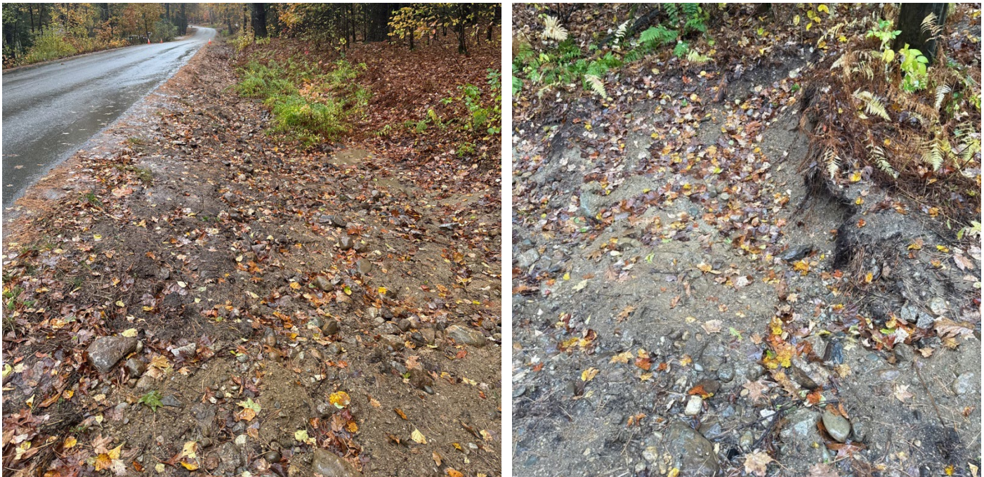
Exposed sediment along the road shoulder with visible erosion gullies (left), and an unstable sediment bank eroded by high-flow conditions (right).
