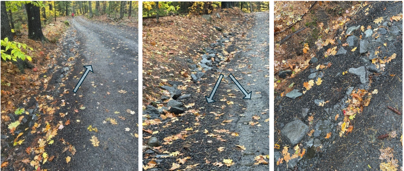
Erosion gullies formed in the road ditch and across the dirt road (left and middle). Road gravel is visibly washed into the ditch (right).
