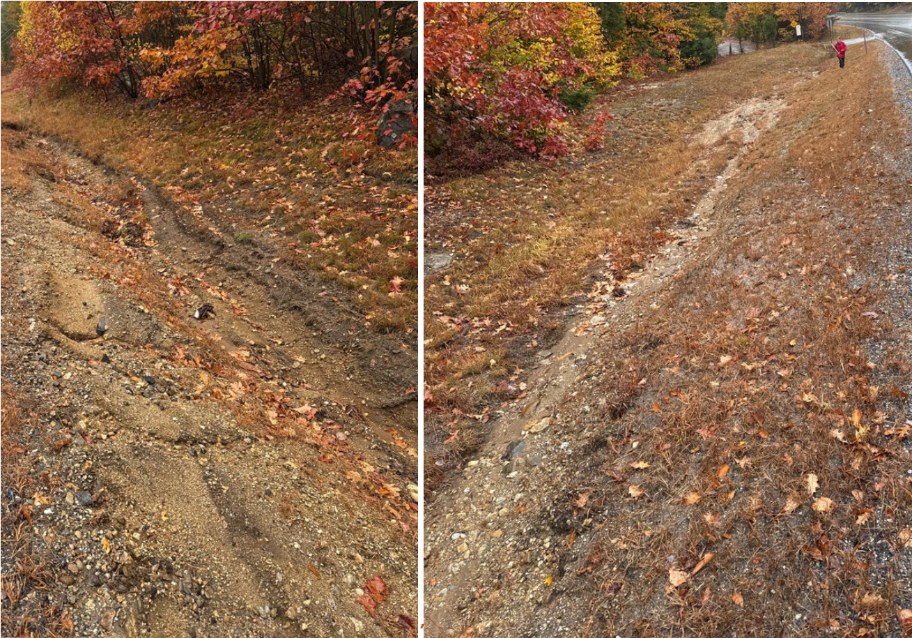
Large erosion gully alongside New Hampshire Route 119. Gully leads to catch basin at the bottom of the hill (right) with a stream down the hill.
